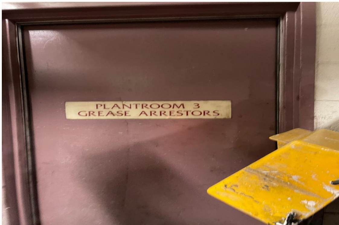
Photograph 6 Grease arrestors, lower ground level
