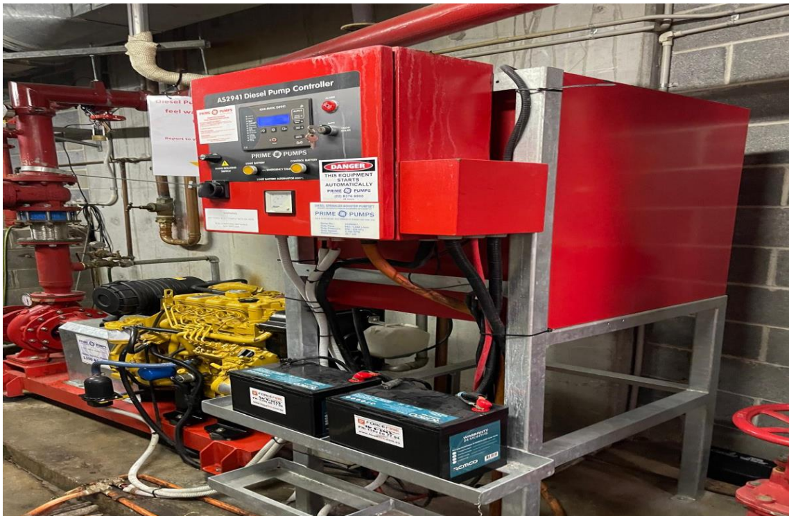
Photograph 2 Above-ground diesel tank within sprinkler / pump room
